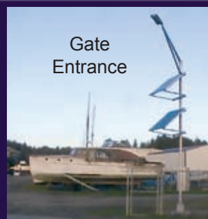
Area Lighting at Night
