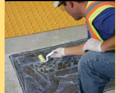
Remove debris from surface. Ensure no moisture is present. Apply TopMark Sealer and Bonder Paste.
